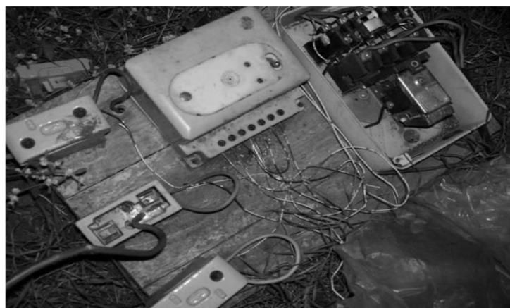
Figure 4: Agriculture pump switchboard placed on the ground.
