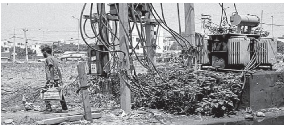
Figure 1: Badly maintained, unsafe electricity transformer.
