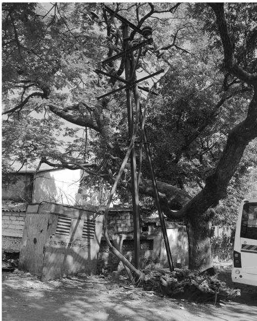
Figure 3: Electricity pole installed very near a tree.
